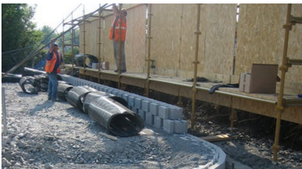
Construction is straightforward and often requires no specialist skills or construction equipment.
