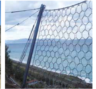
5 Dynamic Rockfall Barriers
