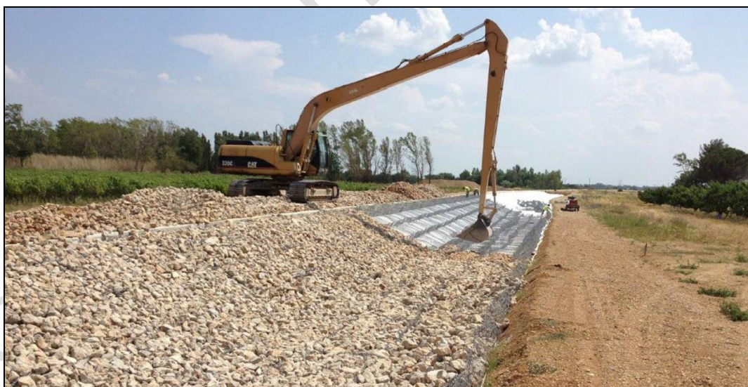
Overview of the different installation phases (1- Geotextile laying; 2- Reno mattresses laying; 3- Reno mattresses filling with stones)
