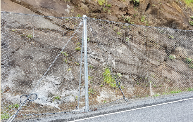
Completed RB100UAF Maccaferri fence system at Whalesback, Kaikoura. Note the use of intermediate post with lateral anchors at both sides of the post.
