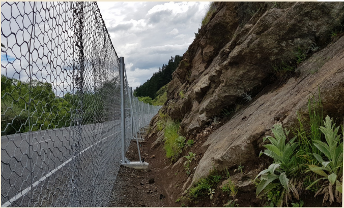
Due to the limited space available between the road corridor and toe of the slope, a fence was the most appropriate option.
