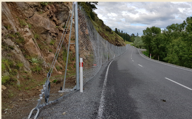
The total length installed was 280 m with a post height of 3.0 m. The fence was installed with an intermediate post at every 50 m section and lateral anchors at both sides.
