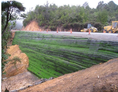
300mm ECT used as facing for an engineered Geogrid Reinforced road support structure.
