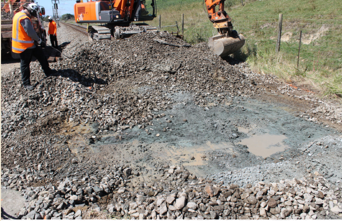
Initial preparation at South end of the site, showing the subgrade condition.
