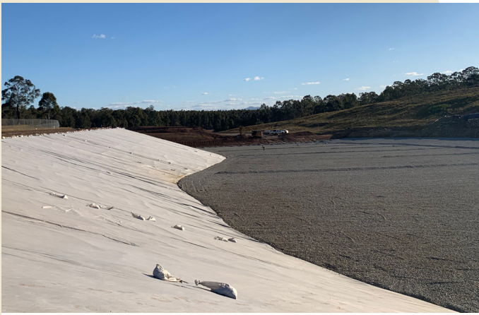
A total of 65,000 m 2 of Bidim A64NF, A84NF and A39NF were supplied and installed.
