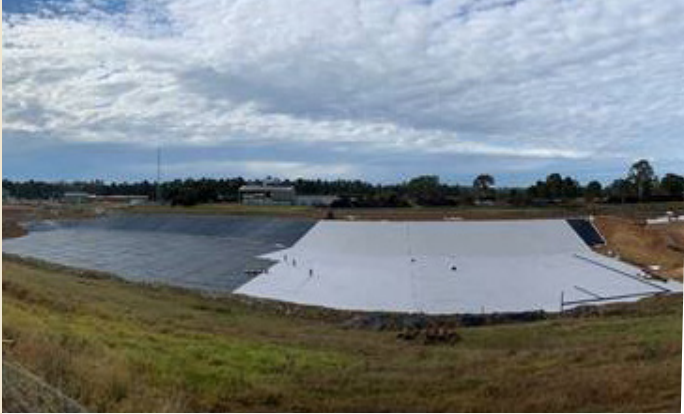
The primary HDPE liner is installed, followed by a layer of bidim A84NF and A64NF.
