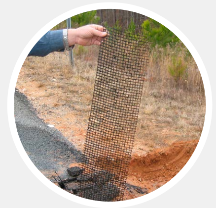
Figure 27: ADFORS GlasGrid carefully removed from the pavement after 5½ years with no damage
