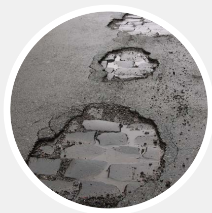
Surfacing failure caused by underlying setts
