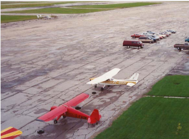
Figure 37: Situation 1992 before treatment
