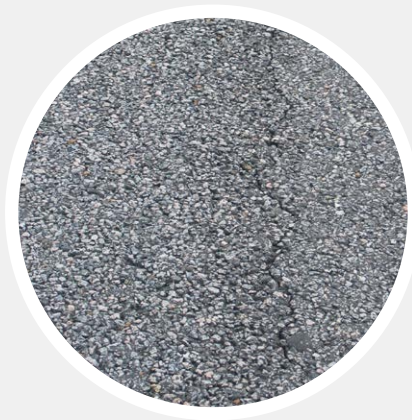
Figure 26: Unreinforced section with cracking
