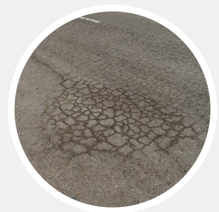
Alligator cracking due to structural failure
