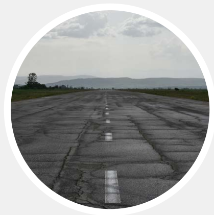
Reflective cracking from concrete bays
