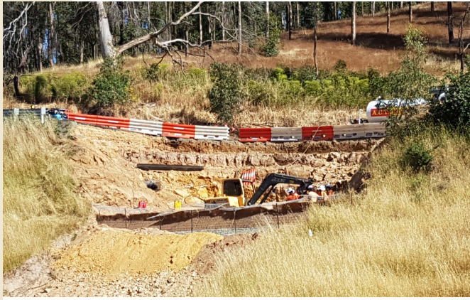
Large road slip for remediation.
