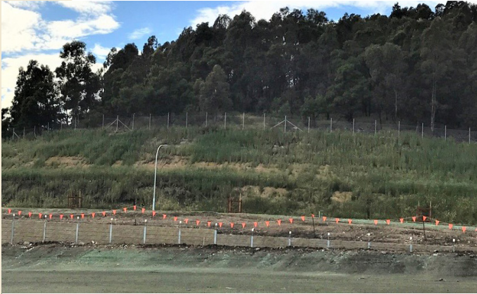
The eroding slope before the installation.
