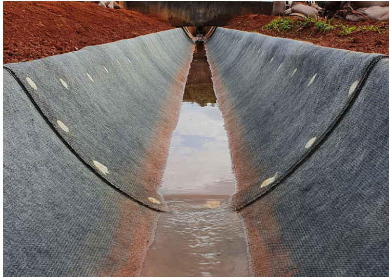
Shot-fired nails were also inserted in overlap joint and sealed with epoxy
