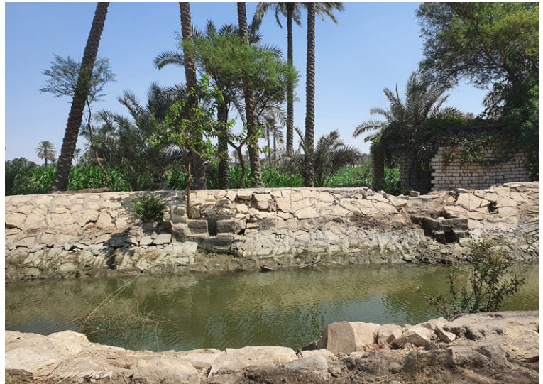
The existing solutions used showing degradation
