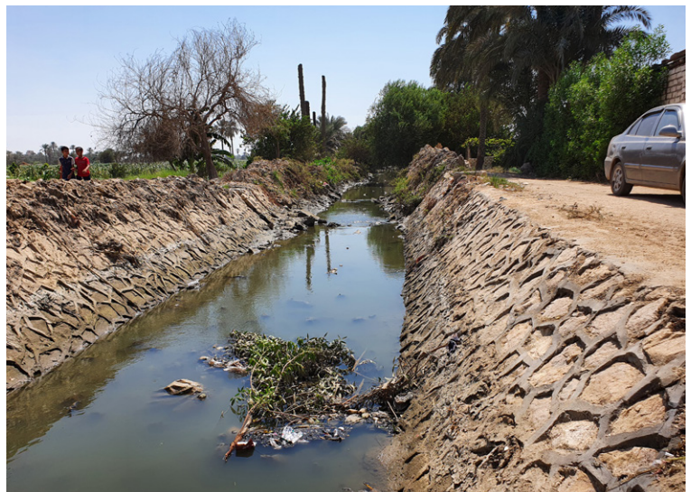
The existing solutions used showing degradation
