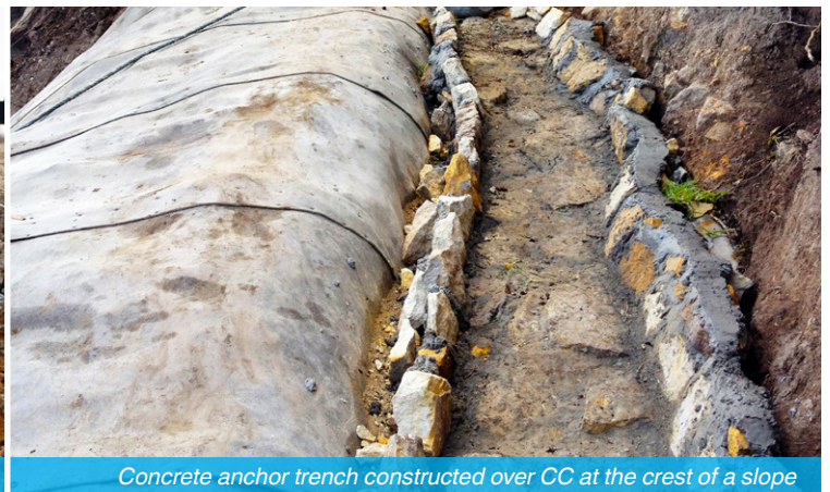
CC fixed at the crest of a slope with ground pegs and anchor trench
