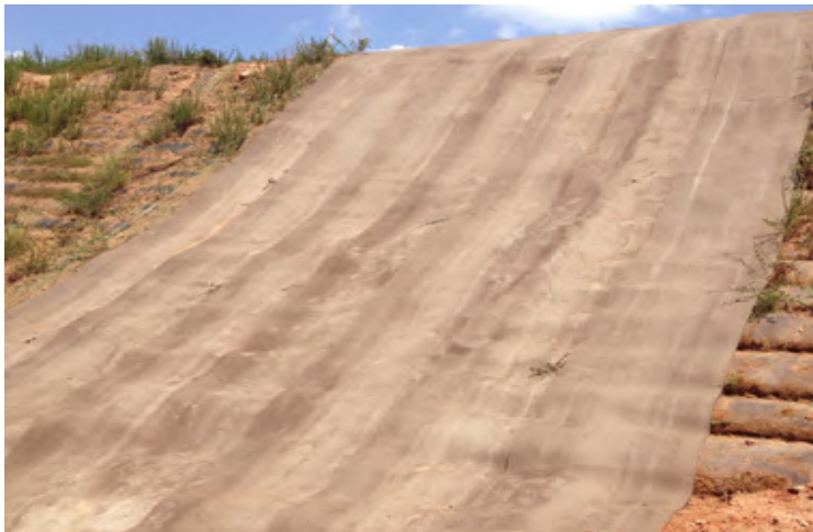
Remediation of Reinforced Soil Slope with insufficient vegetation growth
